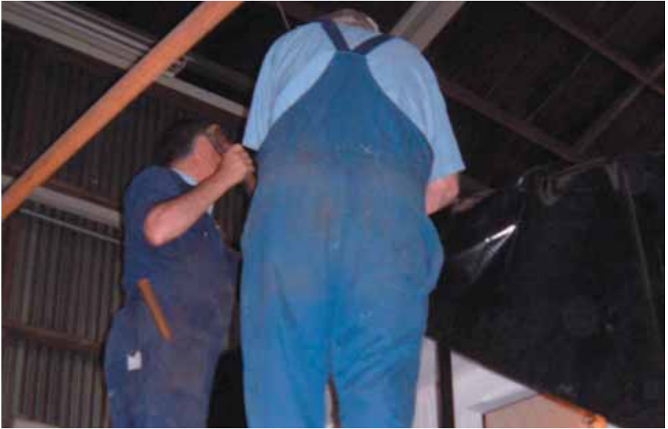
Keith Brown left, with banjo in hand, stretches the roof lining while Graham Inwood drives the tacks. They are nearly finished the whole roof here.
