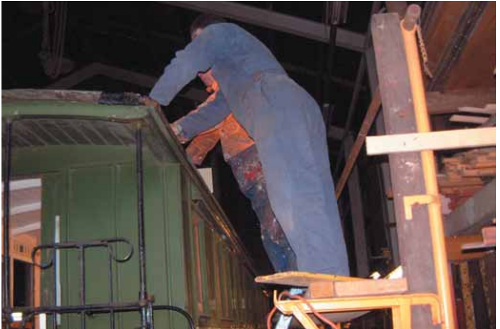
Not to be left behind, Keith Brown and Max Anderson waste no time in finding the best way to rip off the roof covering, (Malthoid.)
